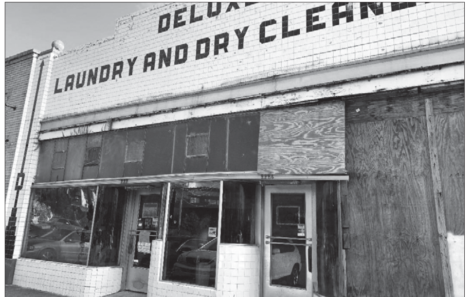
Boarded windows lend to the derelict appearance of the former Deluxe Laundry and Cleaners on Oak Street in Riverside.
