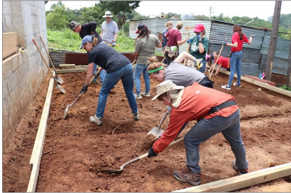
Members of Hendricks Avenue Baptist Church prepare the ground for a foundation.
