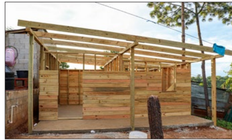
From foundation to tin roof, members of Hendricks Avenue Baptist Church built this house in four days.
