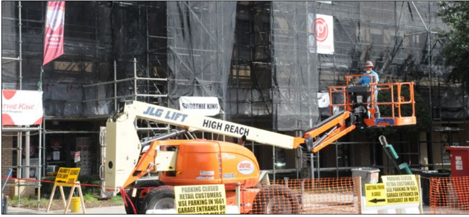
Scaffolding on the Margaret Street side of 1661 Riverside begins at the second story. Construction workers will not have to go inside the shops on the lower floor in order to renovate.
