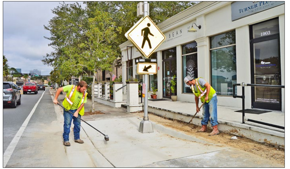
Workmen installed a new pedestrian crosswalk on Hendricks Avenue just across from Turner Plumbing and Bold Bean Coffee House.
