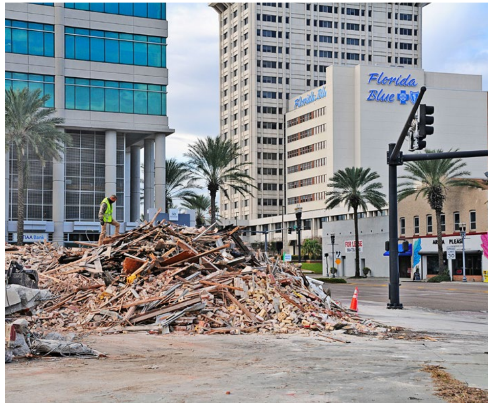
Fire station 5 was vacant for years before the City moved forward with plans to demolish it in order to update the roads leading to a planned corporate headquarters for FIS; no firm plan emerged from the neighborhoods to preserve the station.
