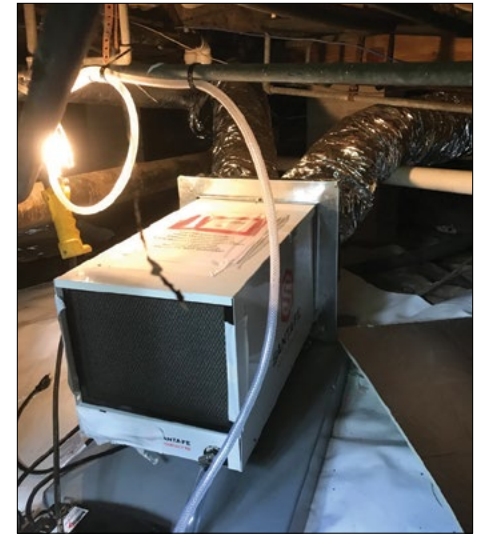
A professional dry system solves Crawlspace problems.
