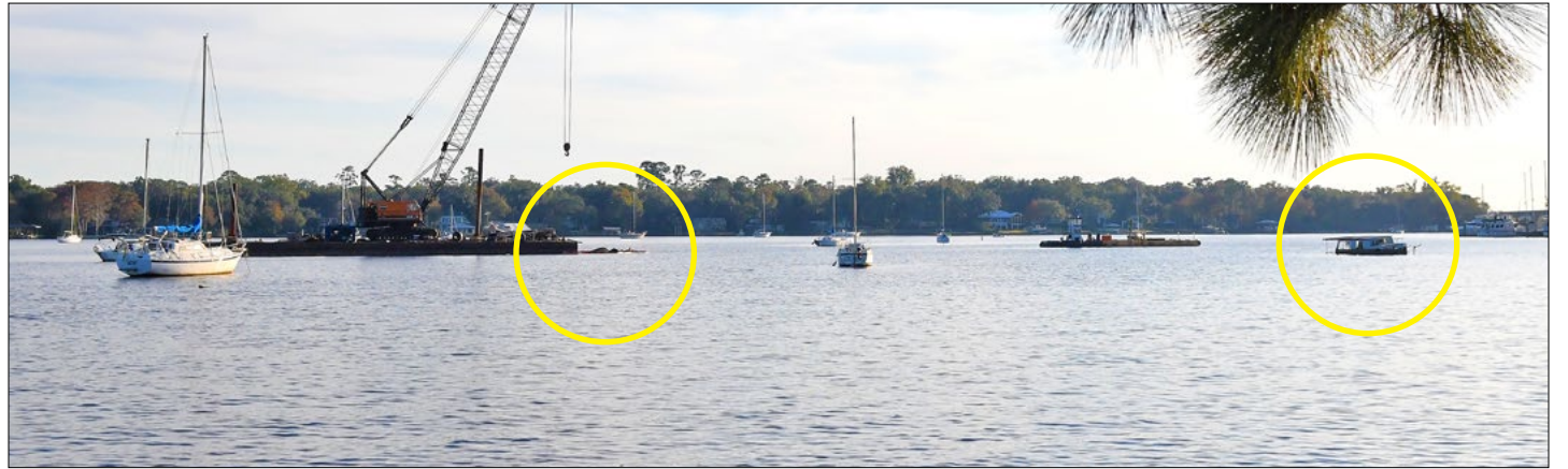
A crane is shown removing a derelict houseboat and floating structure near Stinson Park in Ortega.
