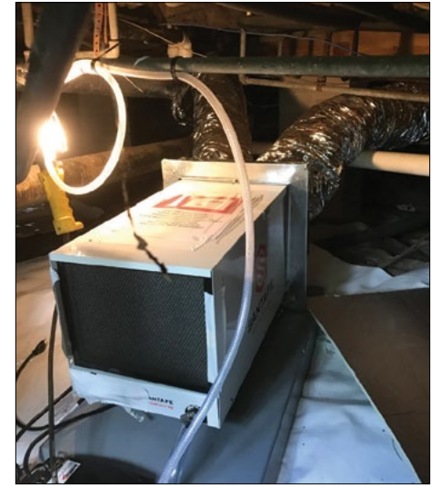
A professional dry system solves Crawlspace problems.
