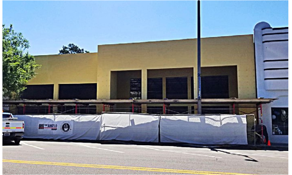
Work on the build out of Southern Grounds Coffee & Co. in the Shoppes of Avondale has been easier because construction workers have not had to compete for parking due to the Coronavirus pandemic.
