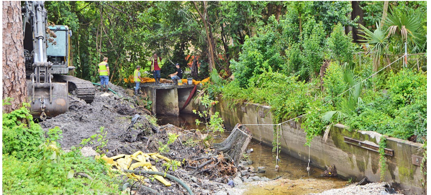
Walls are crumbling along the creek in Willowbranch Park near Olga Place and Willow Branch Avenue.
