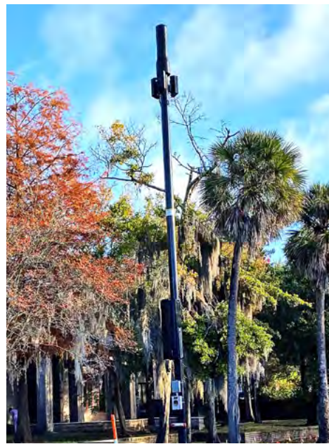
A 5G pole along Riverside Avenue near Copeland Street
