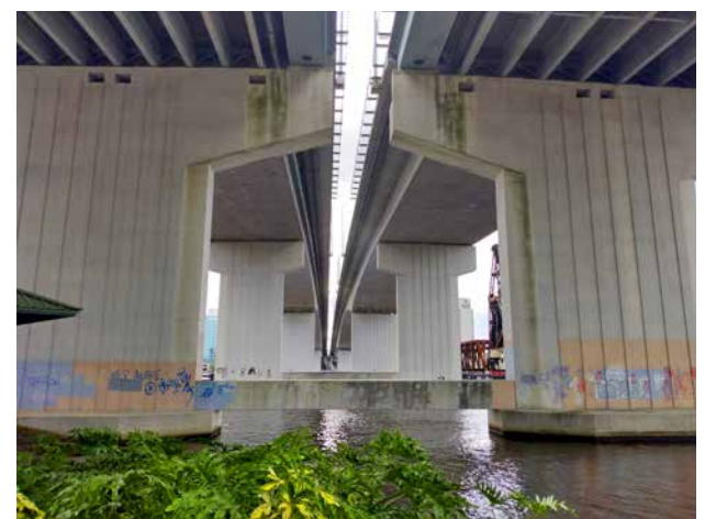
Graffiti covered Acosta Bridge support next to Corkscrew Park on Northbank Riverwalk
