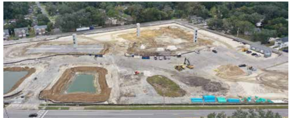
Aerial photo of the site of the former Southgate Shopping Center after demolition
