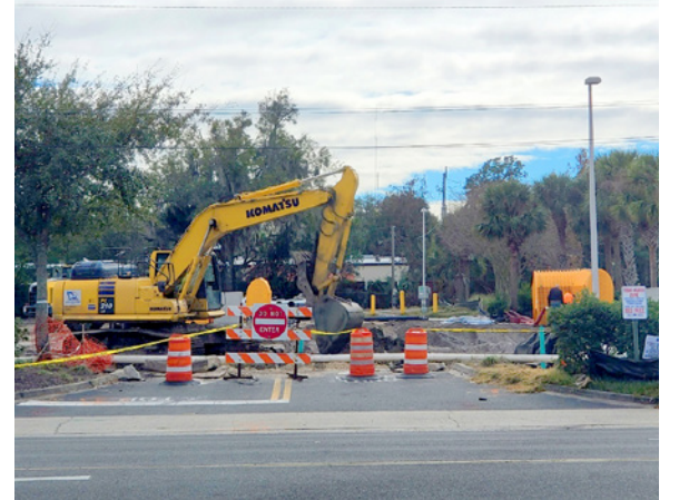
Early January saw the site of the former TD Bank branch cordoned off as excavators worked to clear the site.
