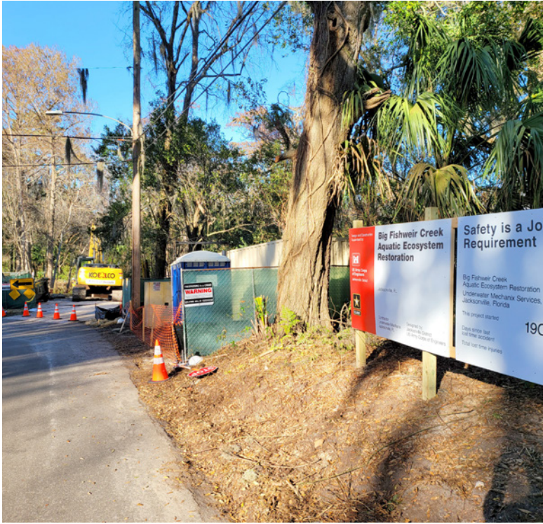
Construction equipment and signage has already been staged for the project to dredge and restore Big Fishweir Creek.
