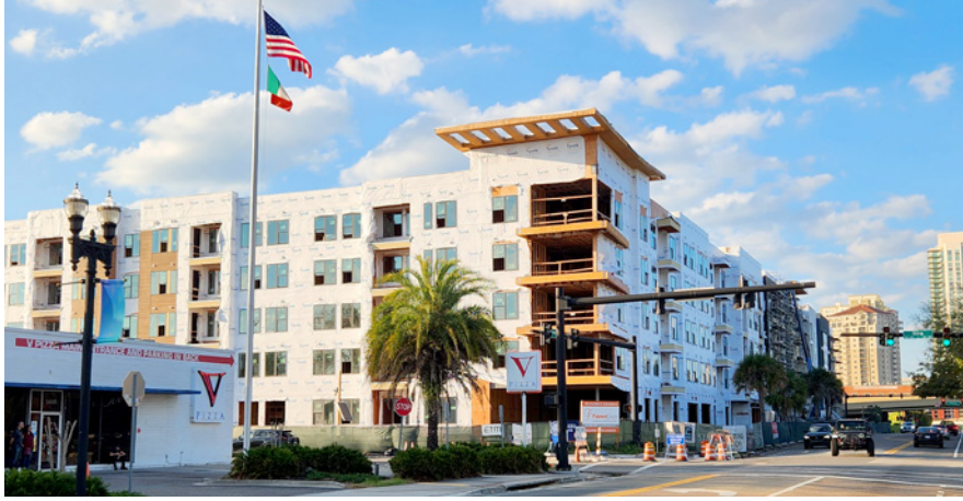
Construction on the Station at San Marco is expected to complete by the fourth quarter of this year.
