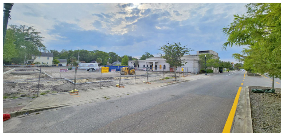
Construction is underway on a reconfigured parking lot for a medical office building on King Street.
