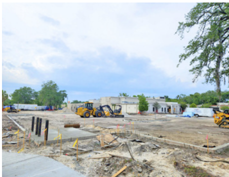
Workers are renovating and retrofitting the property's existing building into a 25,000-square-foot medical office building for women's health.
