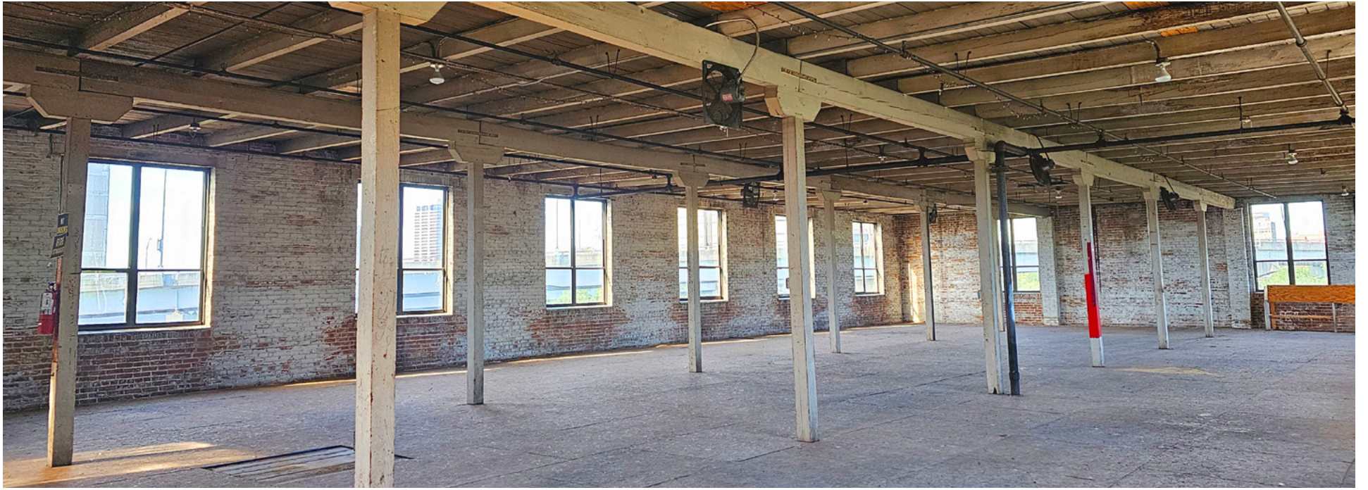
Afternoon sunlight streams through the once bricked-over southwest windows of the Florida Casket Company building as work continues at the Jacksonville History Center.
